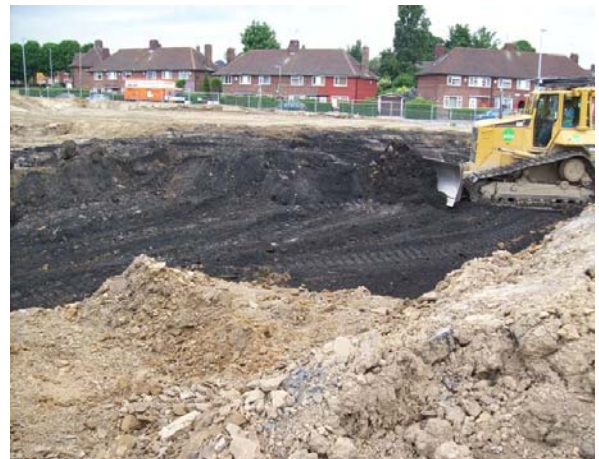
Coal close to the surface being extracted as part of ground works: prevents sterilisation and effective method of remediating unstable ground caused by former coal workings
