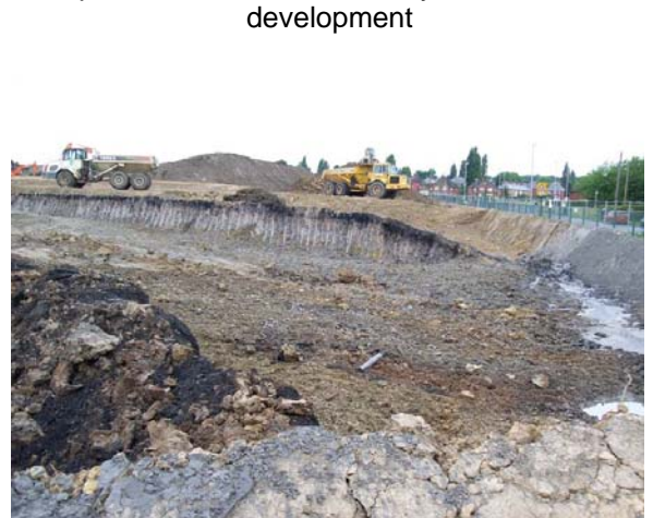
Outcrop of coal close to the surface which would be sterilised without prior extraction and has the potential to cause instability for surface development
