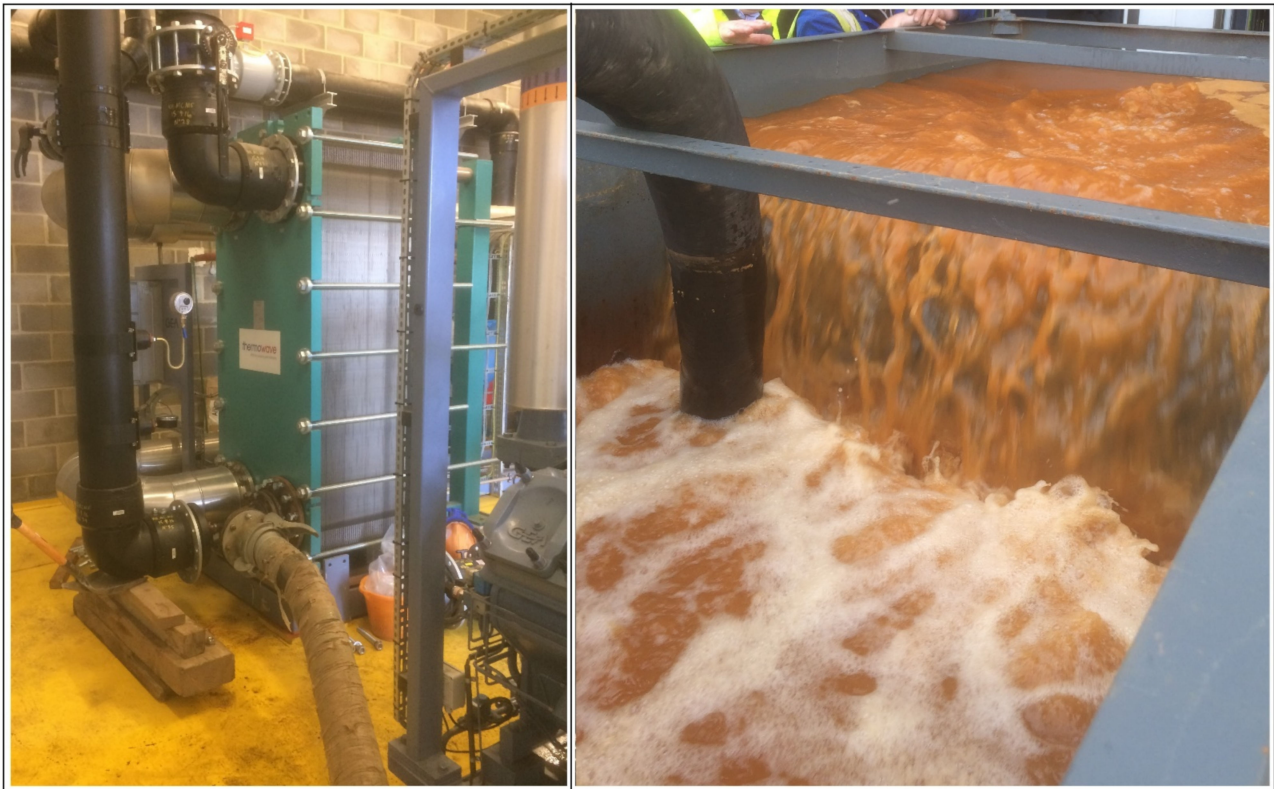
Figure 4. Periodic recirculation of citric acid solution through the plate heat exchanger at Abbotsford Road, Gateshead, UK (left), to remove accumulated ochre (which can be seen in the recirculation tank, (right)). Reprinted with permission from ref. [70]. Copyright 2019 David Banks.
