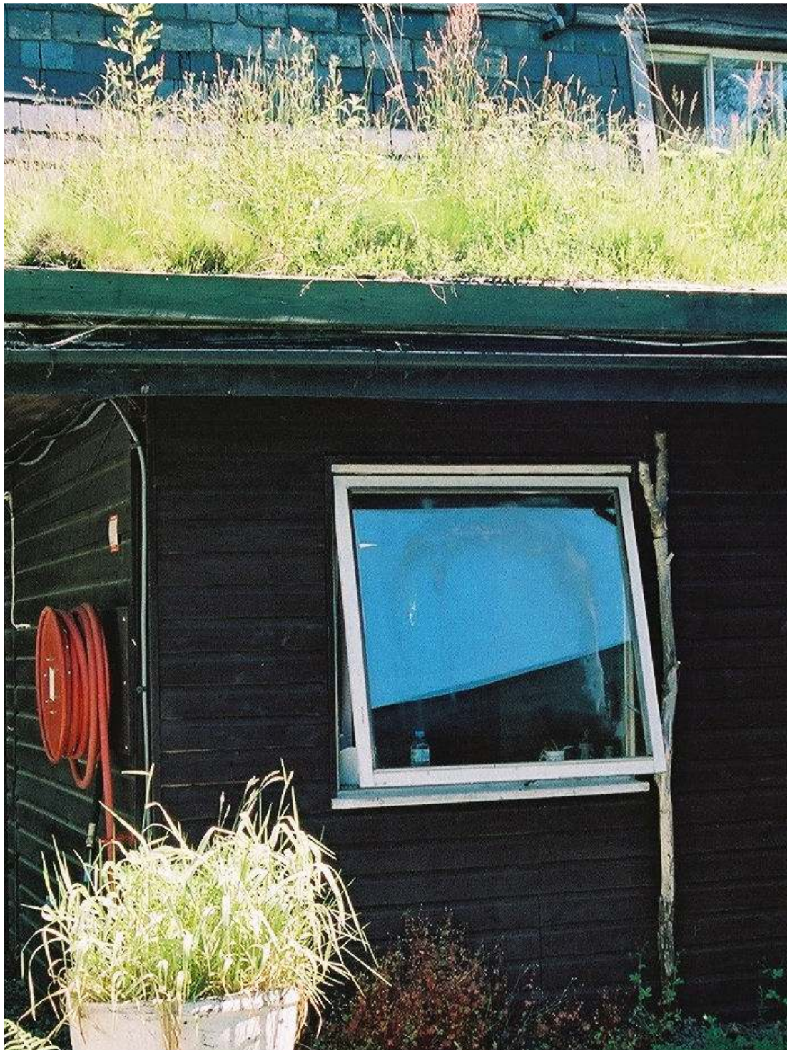
SUSTAINABILITY - 'GREEN ROOF' AND TIMBER CONSTRUCTION FOR EXTENSION. (CENTRE FOR ALTERNATIVE TECHNOLOGY, MACHYNLLETH, POWYS)
