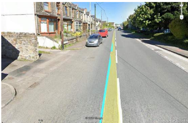
Image 21 – Lack of dropped kerbs and tactile paving at junctions along A48 Pyle Road (© Google Streetview 05/18)
