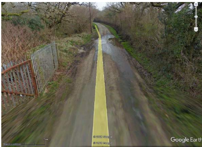
Image 25 – Poor drainage on country lane leading to Waun Bant Road. (© Google Streetview 03/11)
