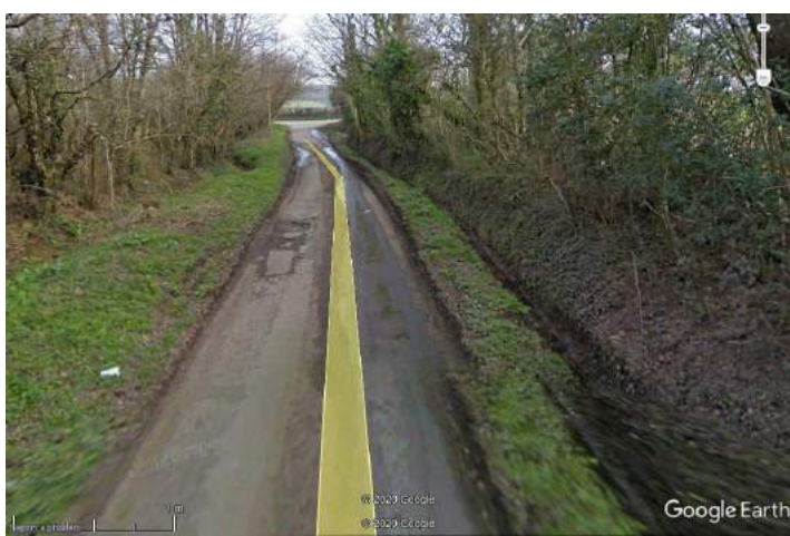
Image 26 – Evidence of vehicle overrun which suggests narrow widths that could intimidate pedestrians/cyclists. Carriageway also in poor state of repair with potholes evident. (© Google Streetview 03/11)
