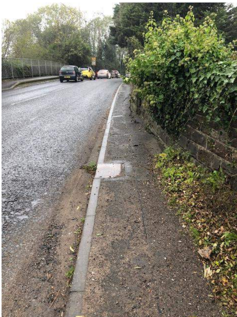
Image 17 – Footways on eastern side of A48 Pyle Road are narrow (Photo: 16/10/18)
