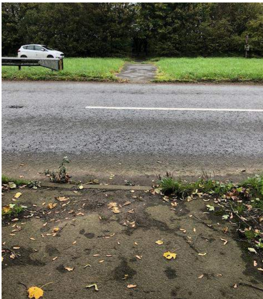
Image 14 – Pedestrian footpath through to A48 Pyle Road is poorly lit, overgrown and narrow (Photo: 16/10/18)
